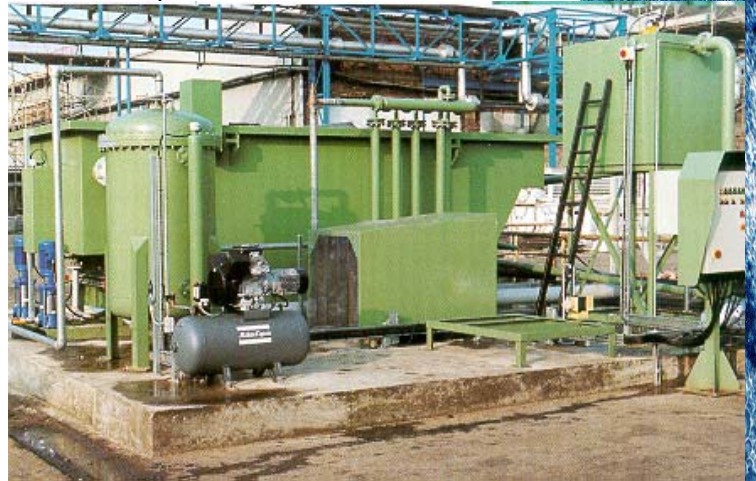
A typical DAF unit, treating oily waste, where quality of effluent containing less than 5 mg/l is required
