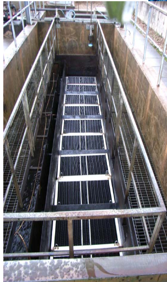
In-ground system with Polypropylene plates housed in stainless steel casings
