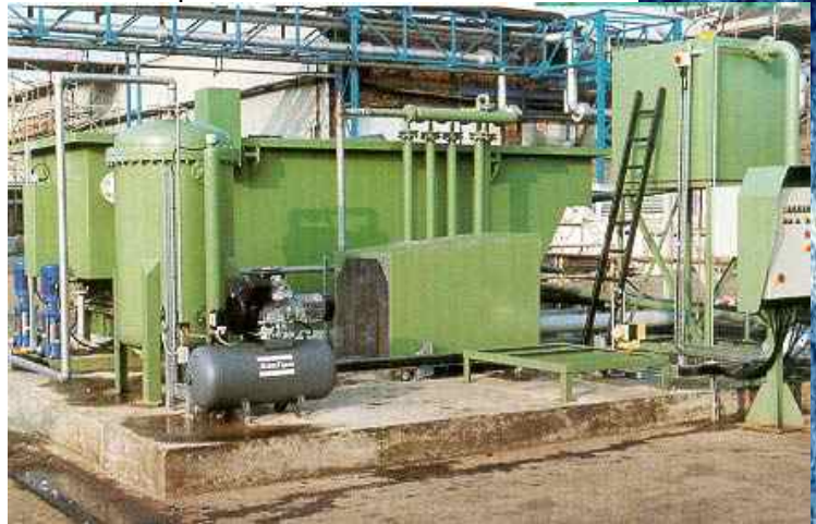
DAF unit, treating oily waste, where quality of effluent containing less than 5 mg/l is required
